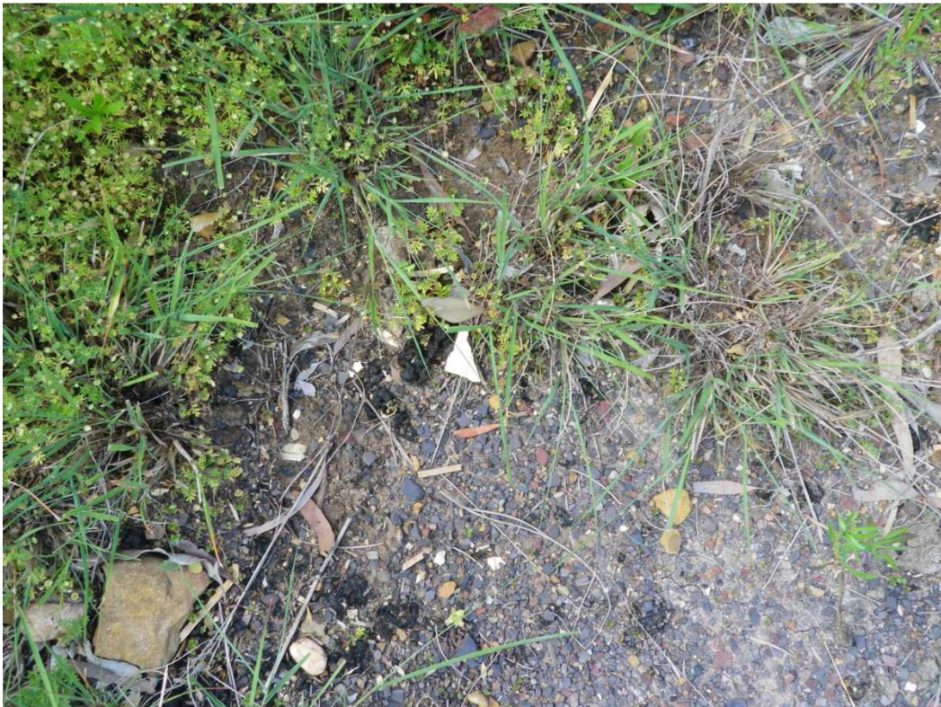
Plate 10 - Fibro fragments noted in old footings in “Old Duck Farm”
