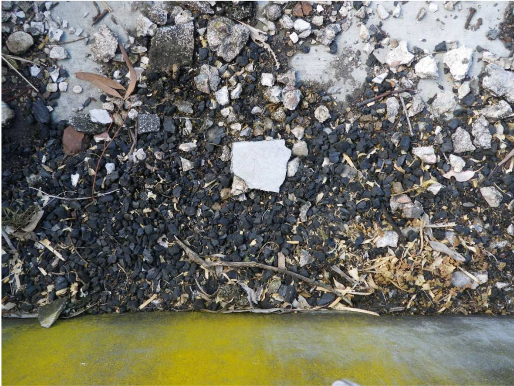
Plate 9 - Fibro fragments noted in old footings in “Old Duck Farm”
